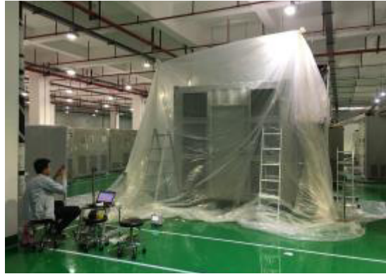
AC Station: Full Load Temperature Rise Test
